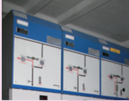
Cell detail of CGM-CGC-24 on Ormazabal PFU-3 transformer substation.
