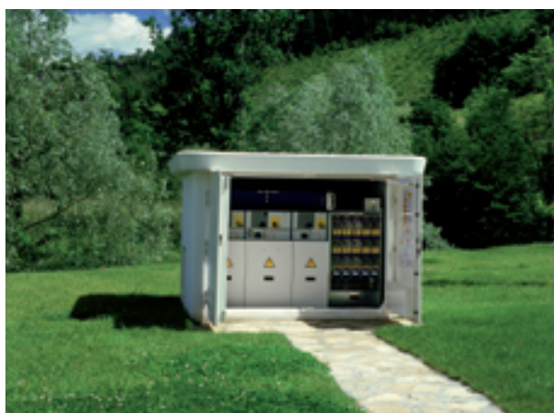
Improved model PFU-3 transformer substation by ORMAZABAL.
